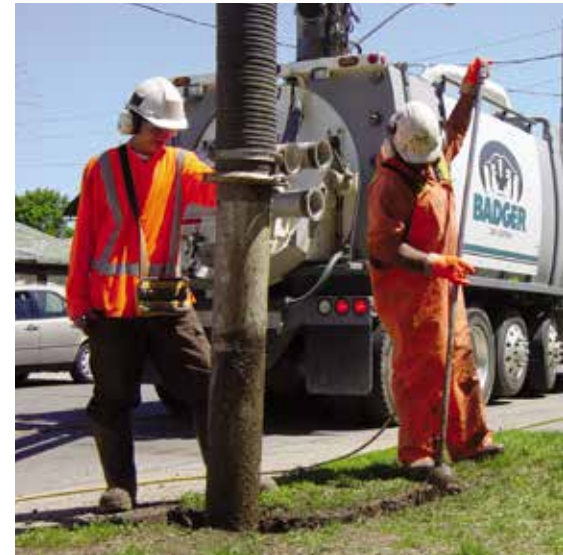
A gas anode service pit.
